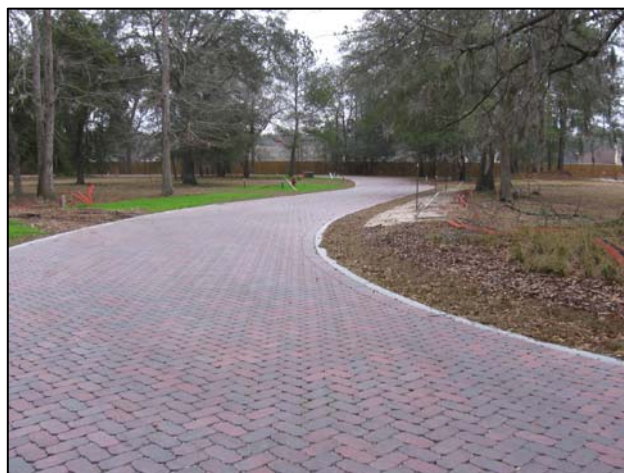
Figure 7.9: Reduced Street Width Used on a Residential Development Site (Source: Center for Watershed Protection)
