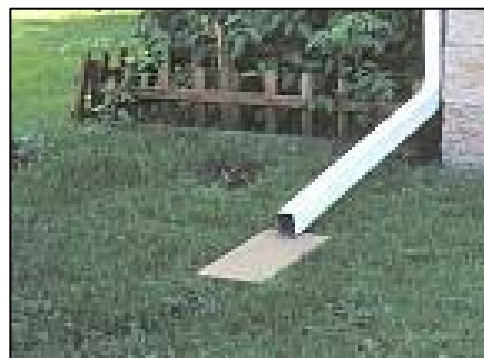
(Source: Center for Watershed Protection)
