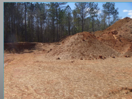
• No sediment barrier • Not stabilized
