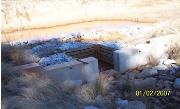
Figure 3. Slotted Board Dam
