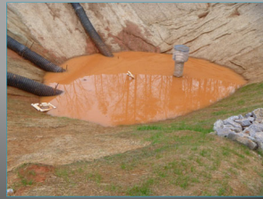
• Damaged - needs repair
