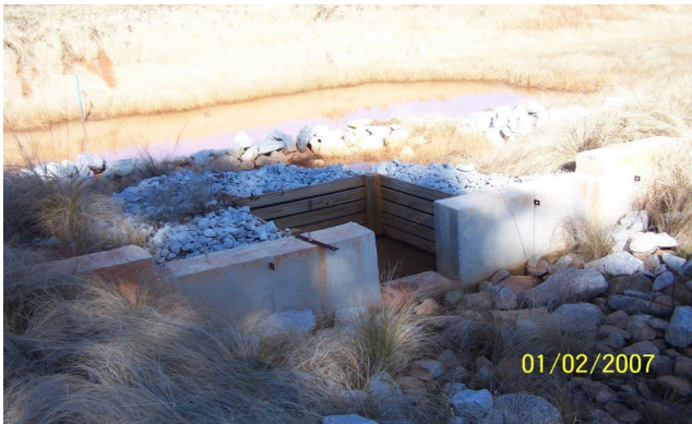
Figure 3. Slotted Board Dam
