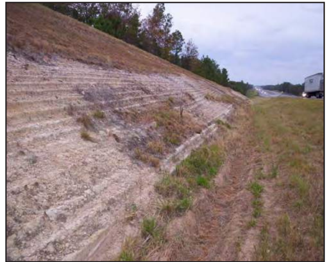
Figure 2.4 - Unstable soil conditions, as on this roadbank, should be avoided.
