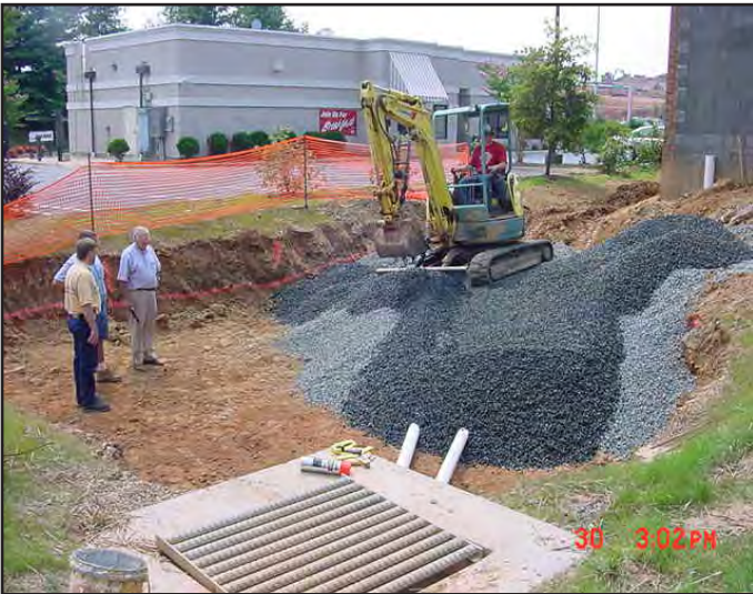
Conversion of a small-scale sediment trap to bioretention. The photos shows adding an under-rain system.
