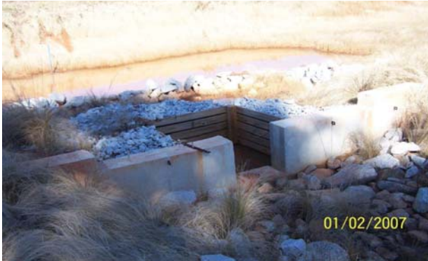
Figure 3. Slotted Board Dam
