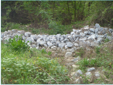
TO BE SHOWN ON THE EROSION AND SEDIMENT CONTROL PLAN 1. Figure 6-24.1, noting rock size as specified in Appendix C. 2. Top and bottom widths.
